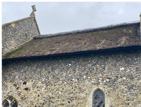
Ingworth, work required to address further deterioration of the thatched roof.
