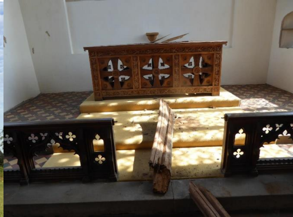
The fallen roof beam
